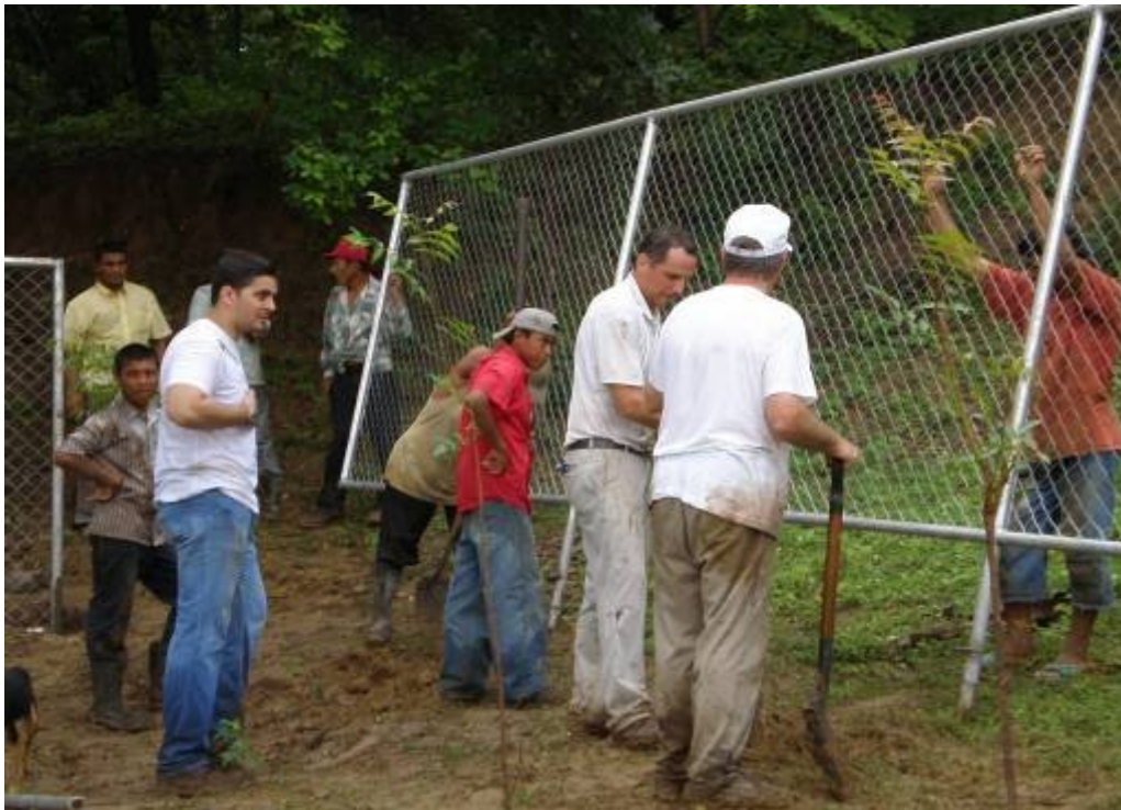
6- Franco, David Slick, David's Son Benjamin and parents from Osneida installing the fence.
